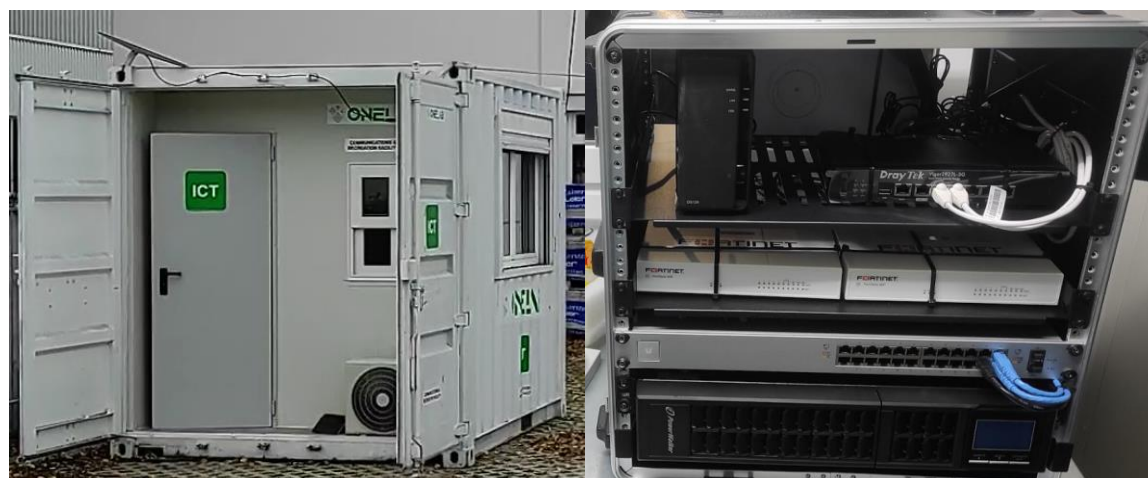
Figure 37 Deployed ICT Enclosure and ICT Module
